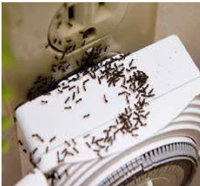
Ants damaging electric infrastructure © Creative commons
